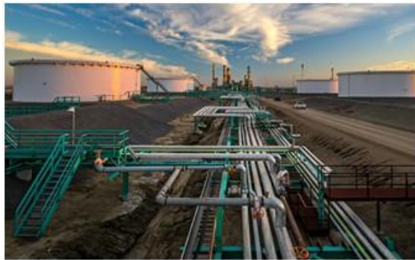
Engineered Platforms for Economic Growth COOP Oil Refinery and Upgrader, Regina
